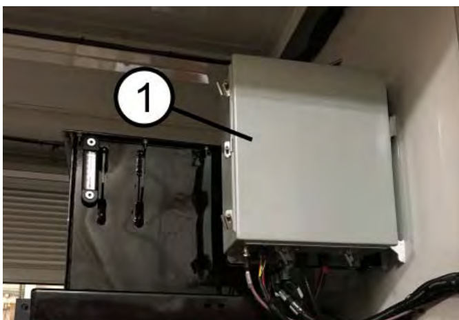
Power Distribution Panel
